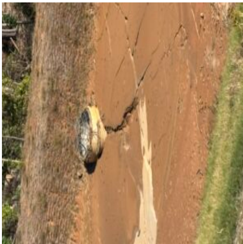
Washed silt in detention pond at Unit 4 phase 2
