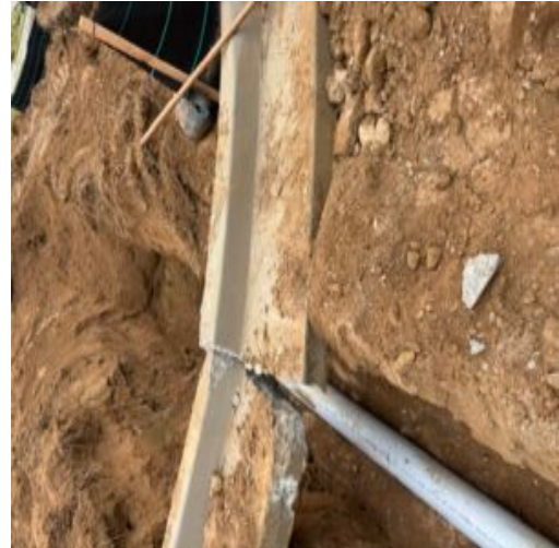
Installing electrical conduit across roadway at Unit 4 phase 2, where curb is severely damaged.
