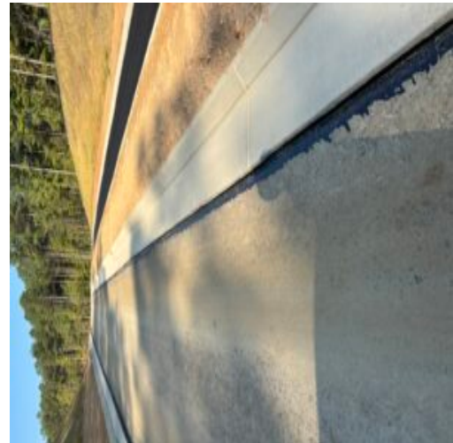
Liquid tack observed at curb lines
