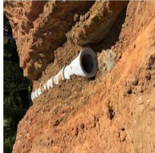
36" rcp between FO -STHW and OCS
