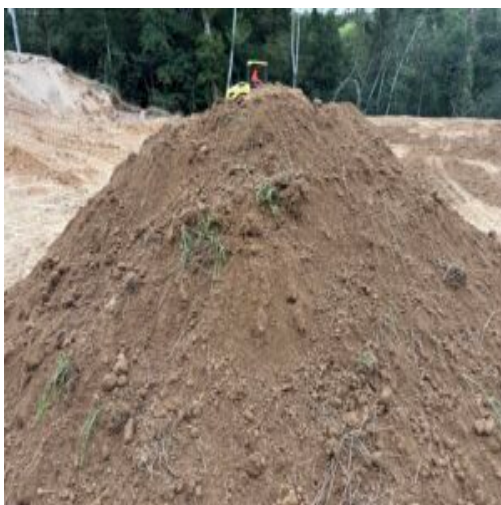
Backfill used on bridge before organics removed
