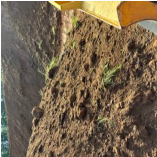
Clipped materials with lots of grass not recommended for structural fill placement
