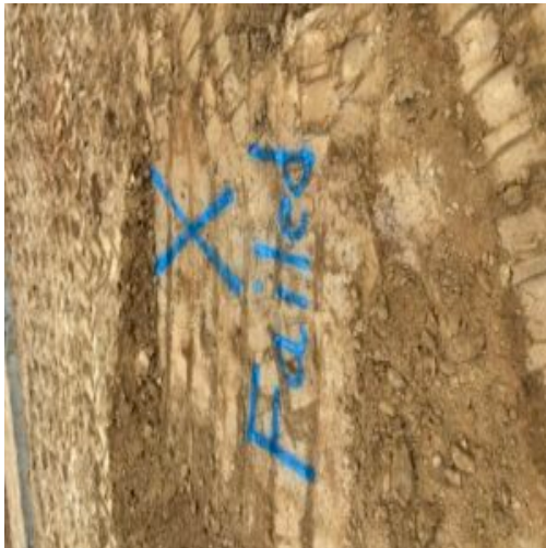
Performed density tests all areas failed
