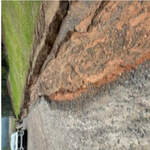
Eroded curb line
