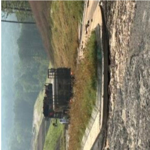
Washed erosion at parkway
