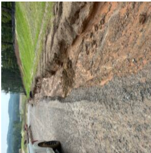
Eroded areas at curb line
