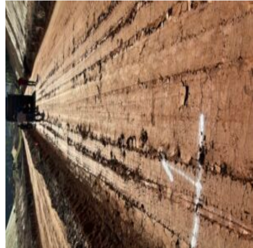
Moderate areas with scabbing painted for repair
