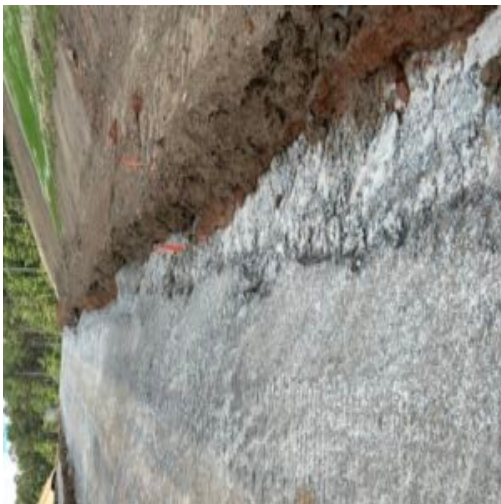
Eroded sub base stone at Nature Walk curb line between sanitary sewer manholes #12 and 13
