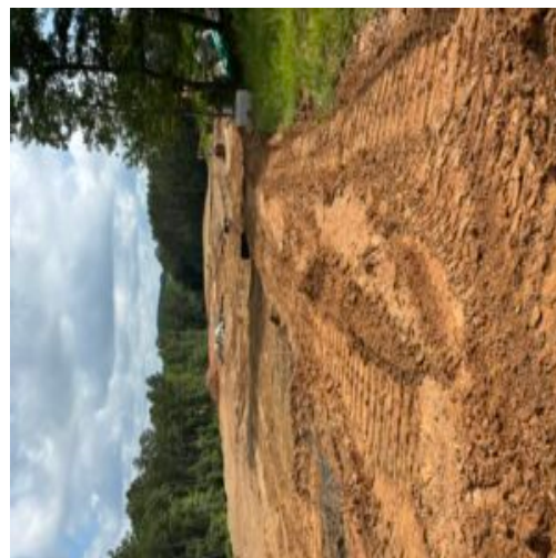
Severe erosion conditions at Seven Hills phase 13
