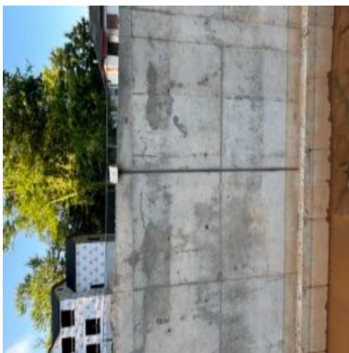
Vertical hairline crack
