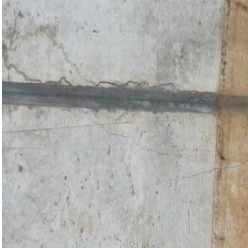
Vertical hairline crack
