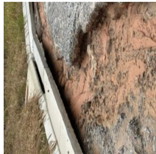
Erosion at existing poured curbing
