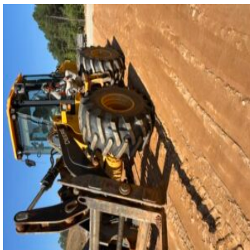
Additional traffic from sub contractors rutting sub grade
