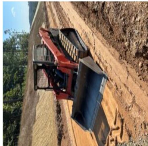
Blading down ruts and scabbing from additional traffic from sub contractors
