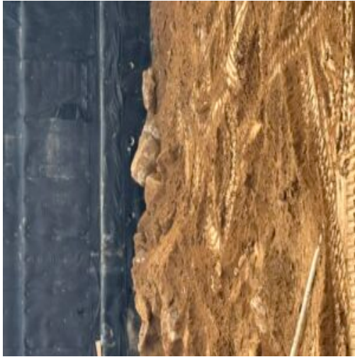
Backfill at westside bridge abutment showing large rocks at wall. The contractor was reminded that no large rocks are required within ten feet of the wall.
