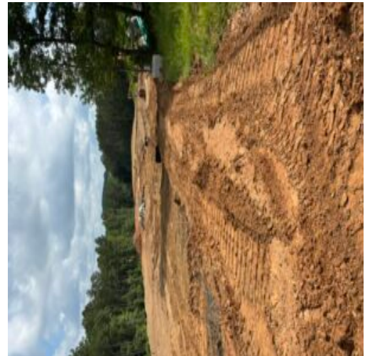
Severe erosion conditions at Seven Hills phase 13
