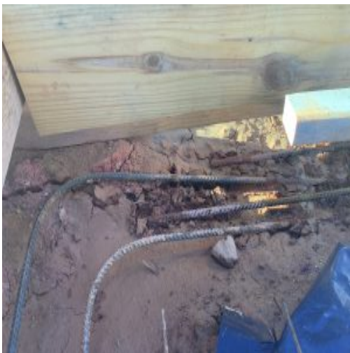
Lot 8 Missing Rebar Ties
