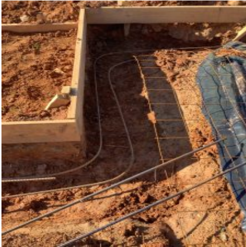
Lot 9 Rebar not aligned with Footing
