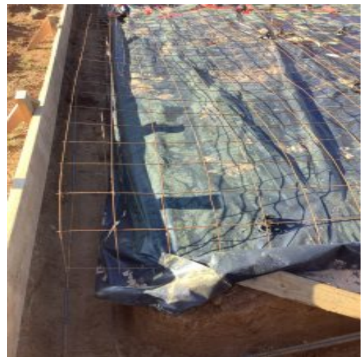
Lot 8 WWR needs trimming
