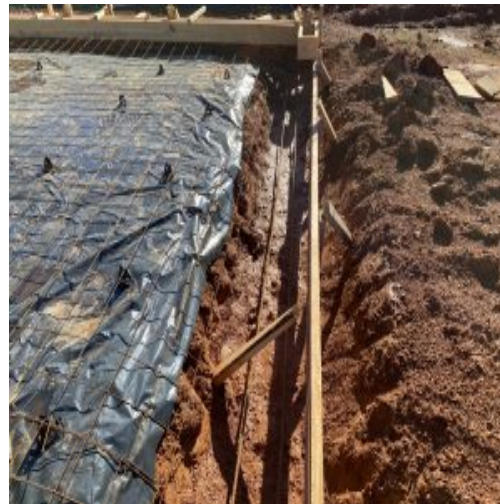
Lot 6 Footing (Heavy saturation) requires “de-mucking”
