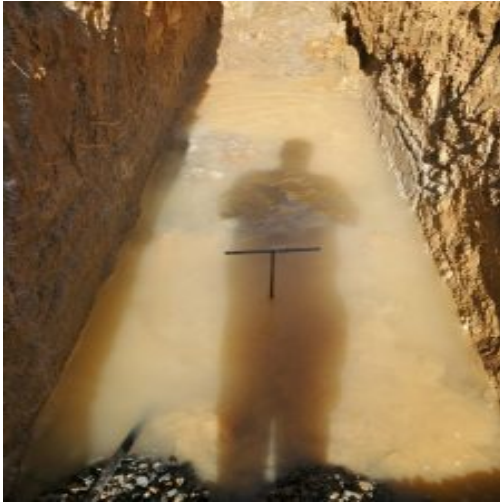
60 LF north of MH-CA22 (water)
