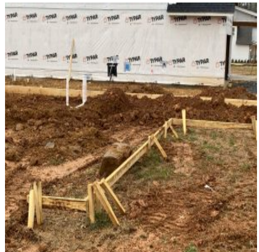
No Rebar/ No Footings
