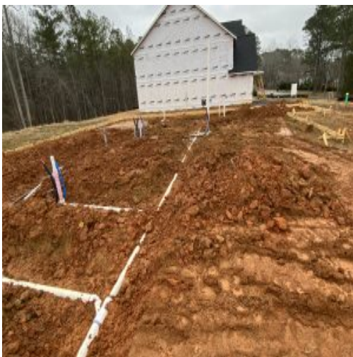
No Rebar/ No Footings
