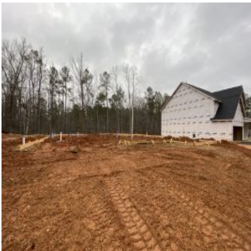
No Rebar/ No Footings
