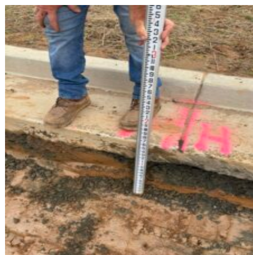
Showing depth of undercut
