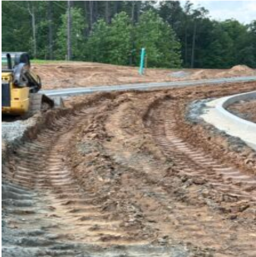
Existing subgrade conditions at roadway
