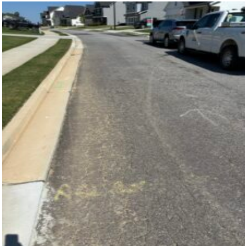
Observation of existing asphalt conditions at Mountain Ash lane with recommendations to use PermaFlex seal coating on cracked surfaces.
