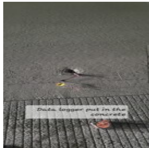
Picture showing how the data loggers installed at specific sites.
