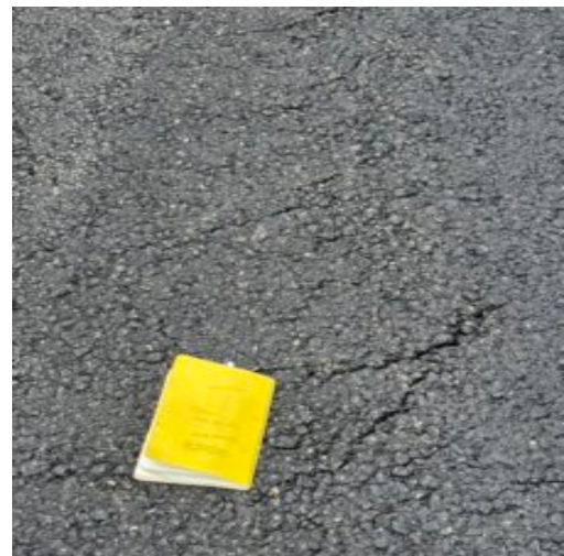
Moderate cracking at Phase 1B
