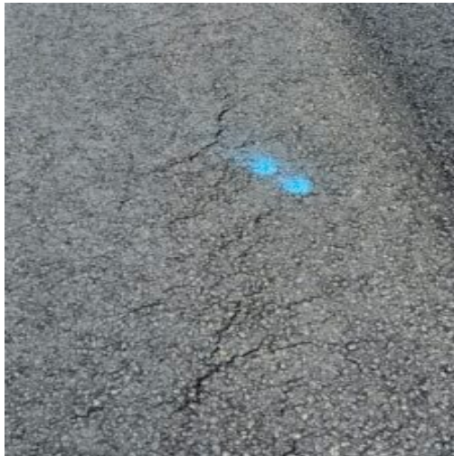
Moderate cracking at Phase 1B
