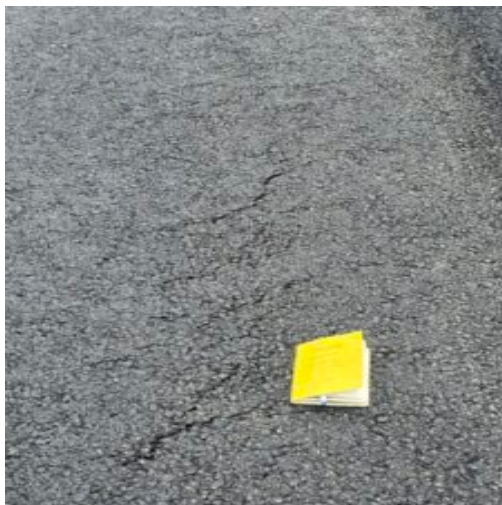
Moderate cracking at Phase 1B
