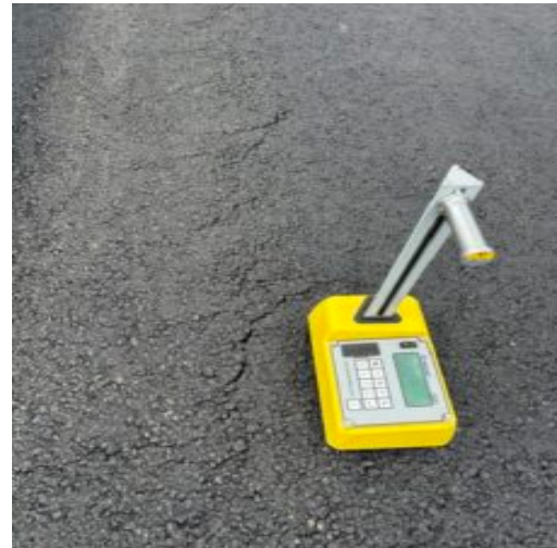
Density check with cracking
