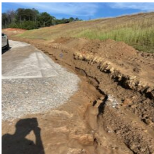
Gullies at curb line after rain event
