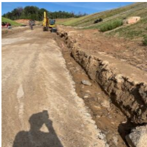
Washed gullies at curb line
