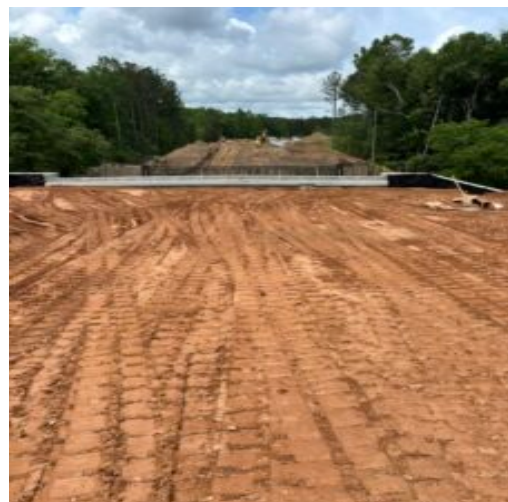
Recommended subgrade repair at crane pad
