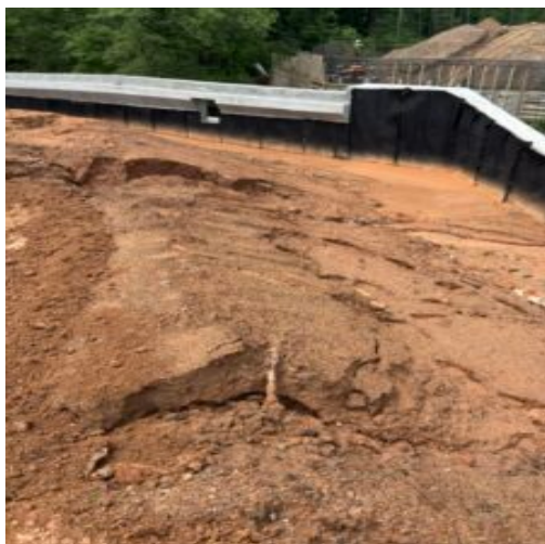
Erosion at wall backfill
