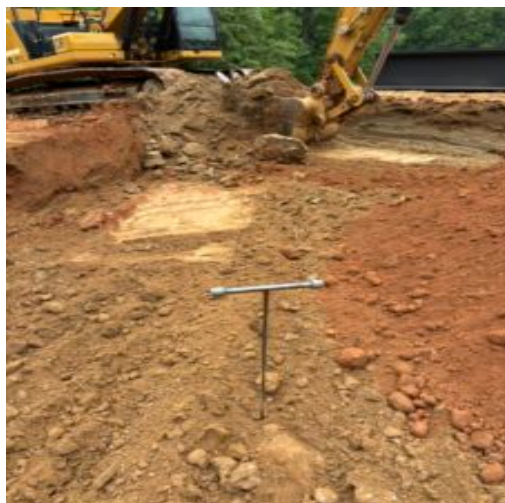
Probing undercut area at crane pad
