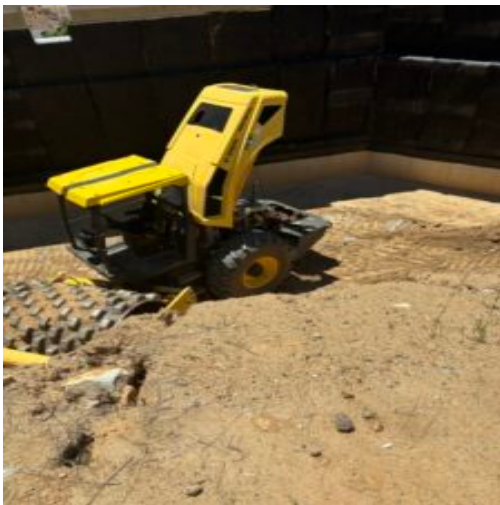
Beginning backfill at wall with equipment failure
