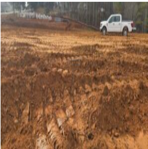
pumping area addressed by contractor
