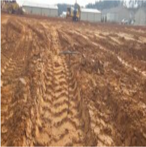
pumping area addressed by contractor
