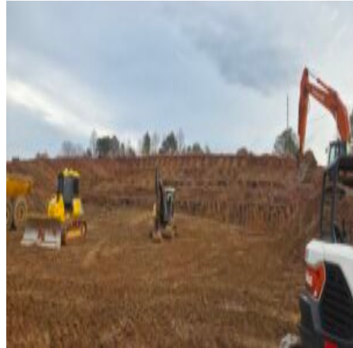
cut area above connexes at main entrance
