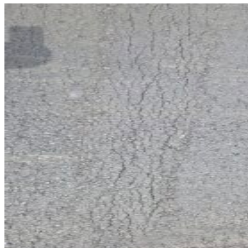
cracking on taxiway
