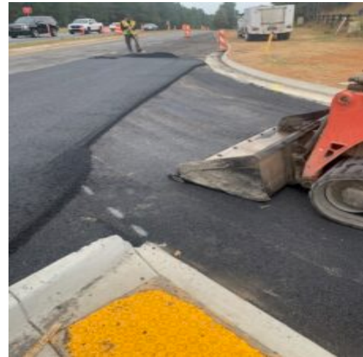
Remaining area wasn't completed with topping mix at exit lane.
