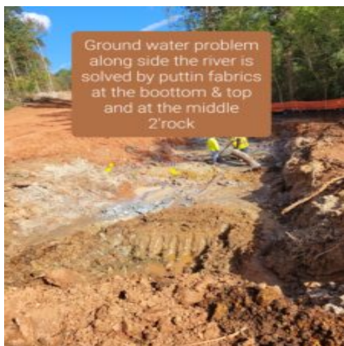
Location showing groundwater problem and fixed by fabric and rock
