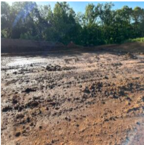
Area adjacent to detention pond requiring remediation.
