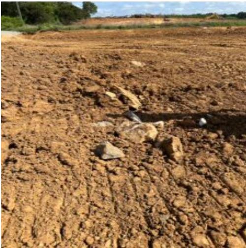
lots 95,96,97 affected area (since covered with soil)
