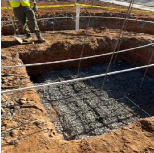
Unable to perform Bering pressure testing due to rebar and 57 stone already in place.
