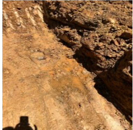
retaining wall footing with water intrusion
