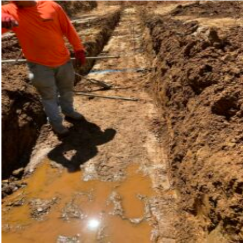
retaining wall footing with water intrusion
