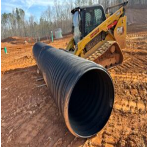
36 inch black corrugated storm drain
