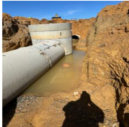
AI4 RCP and corrugated pipe
