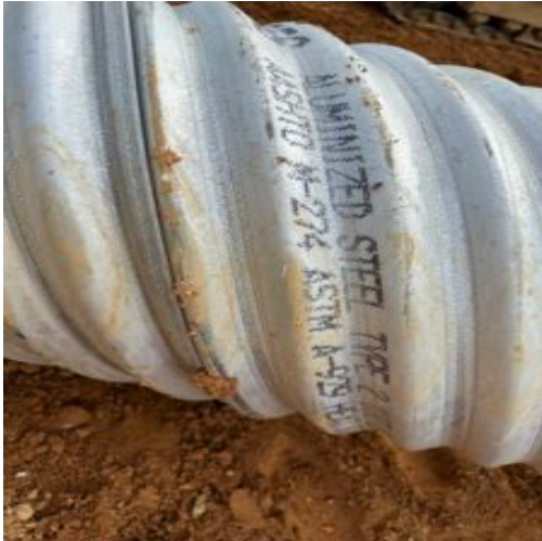
Metal corrugated storm drain pipe
