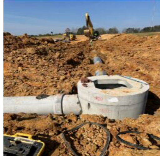
Storm drain AH3
