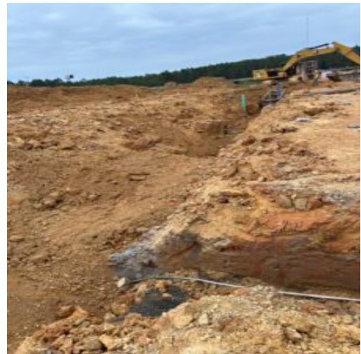
Sanitation pipe with approximately 4-5 foot lift
