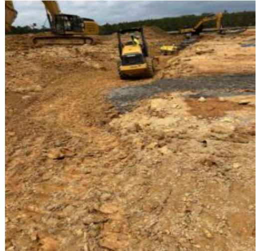
between AH5-AH6 storm drain
