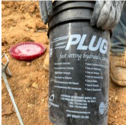
Used instead of gaskets on 2 storm drain pipes E2-E3
