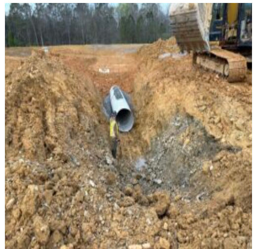
storm drain BA1-BA2
