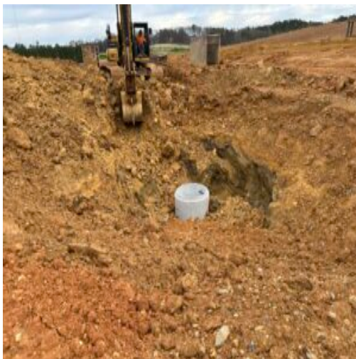
sanitation sewer manhole
