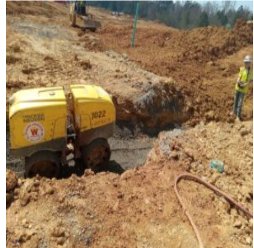
Area 1 Lateral Sanitation Pipe going under road
