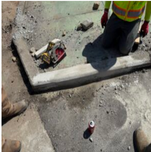
Curb repair area 1
