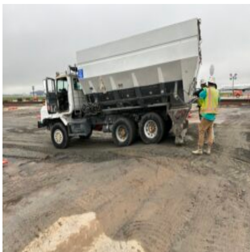
Cement truck issues
