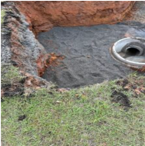
High moisture area with 89 stone after soil removal at A4
