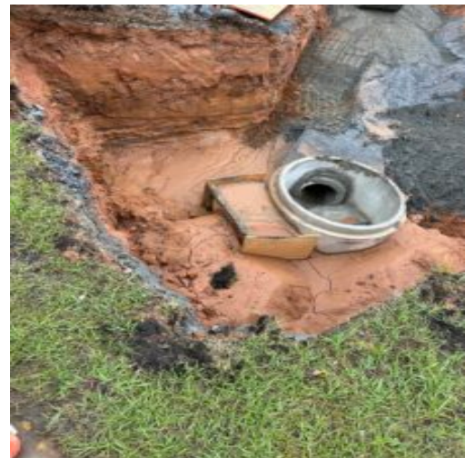
soil with high moisture content/request for removal at A4
