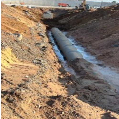
Wet and inundated soils between I3 and I4 structures.
